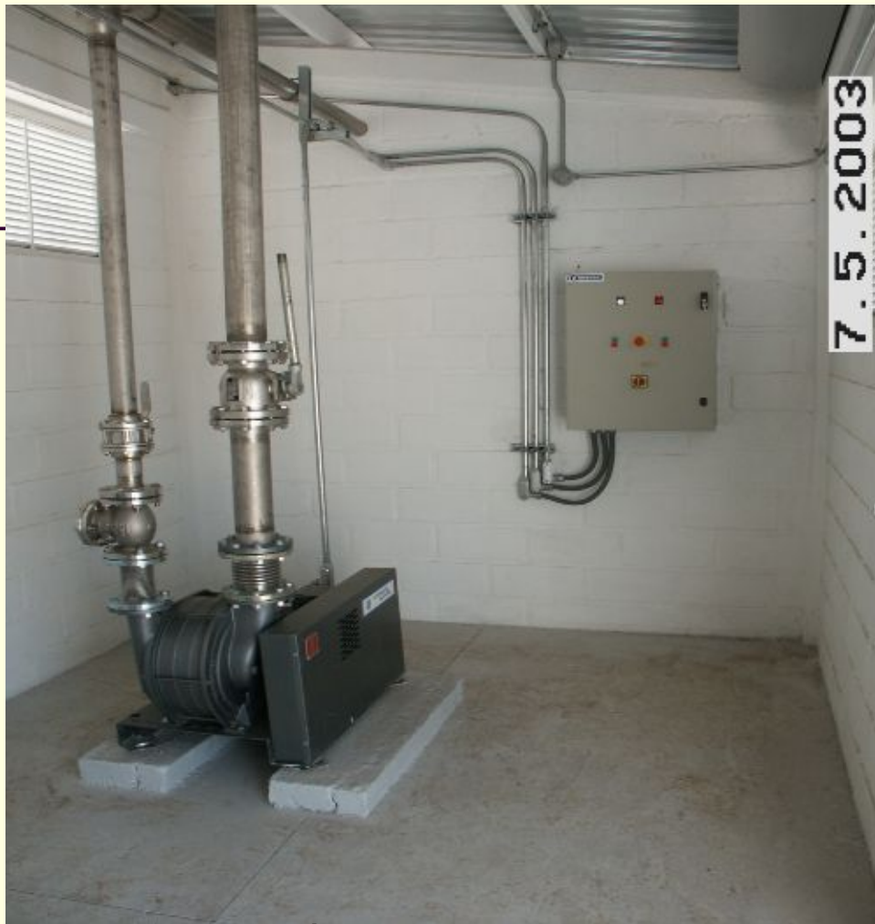
Automatic pressure system
